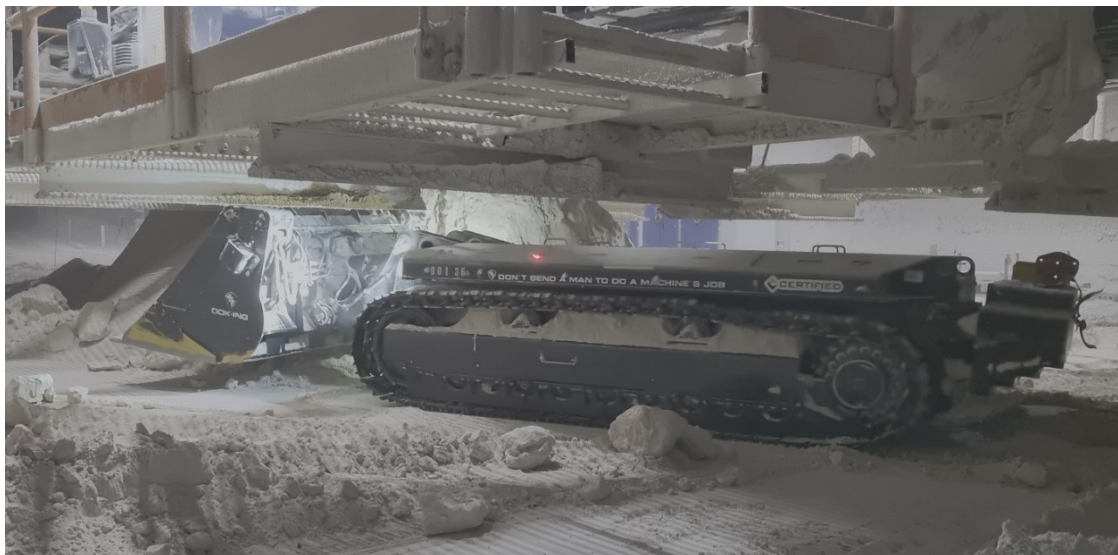
Slika 1 XLPD cleaning under conveyor belt
